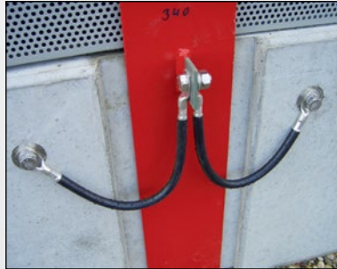
earthing terminals at base elements
